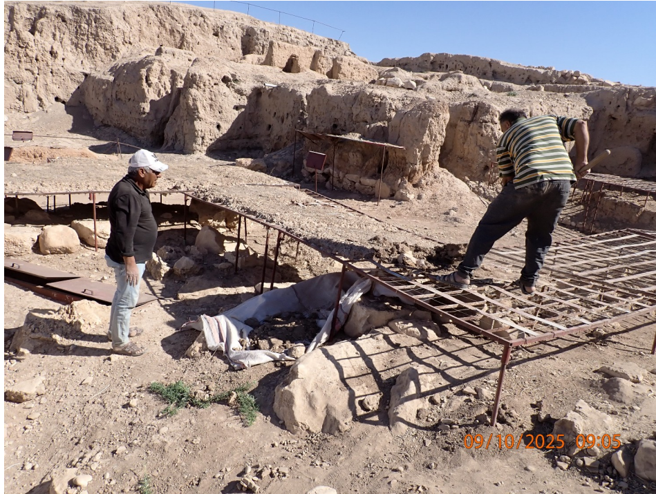
Fig. 11: Removal of the fragile and deteriorated mud plaster
