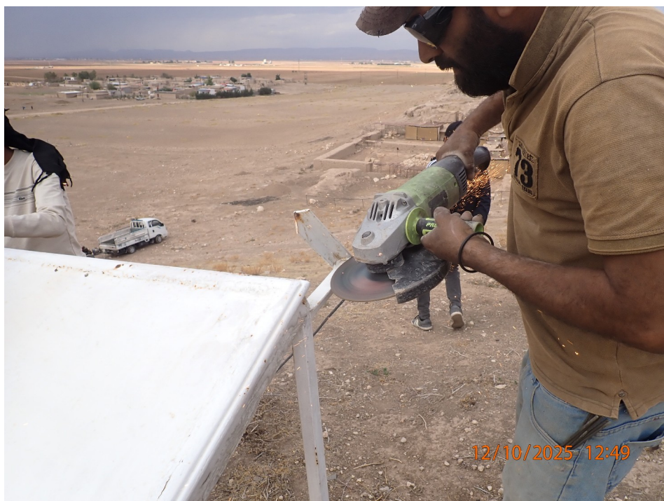
Fig. 6: The cutting of the iron rod that prevented the cover from lying flat
